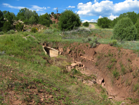
Poorly designed culverts and road drainage systems contribute to erosion and ecological degradation throughout the Basin.
