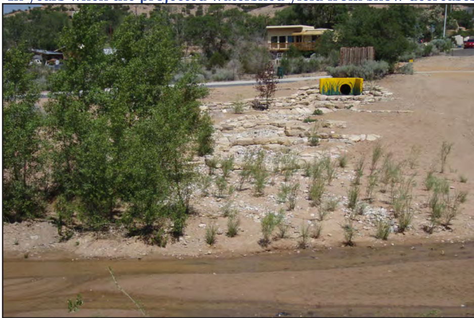
The completed Calle Don Jose drain. Stormwater runoff flows from the neighborhood in the background. Photo by City of Santa Fe.
