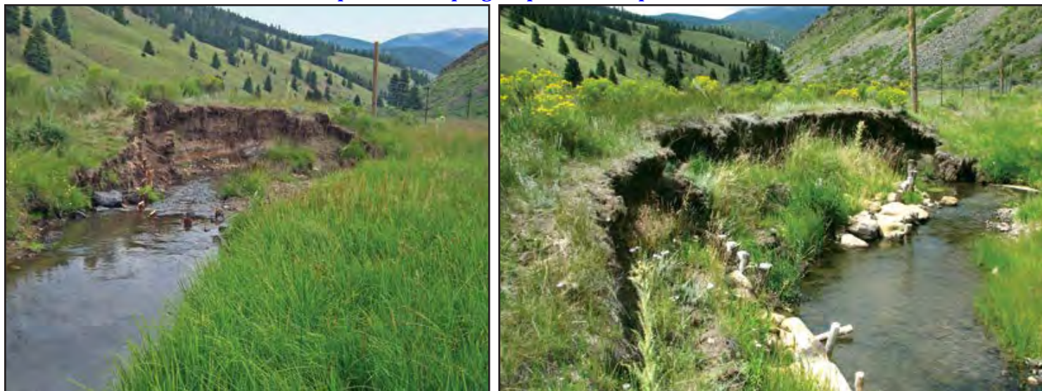
A cut bank on Comanche Creek before treatment (left), and after installation of post vanes (right).
