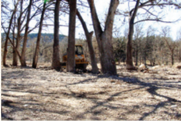
Disturbance with heavy equipment along the banks for floodplain will often result in large additions of sediment to the channel, which disrupts the balance. Photo courtesy of Sky Lewey, Nueces River Authority
