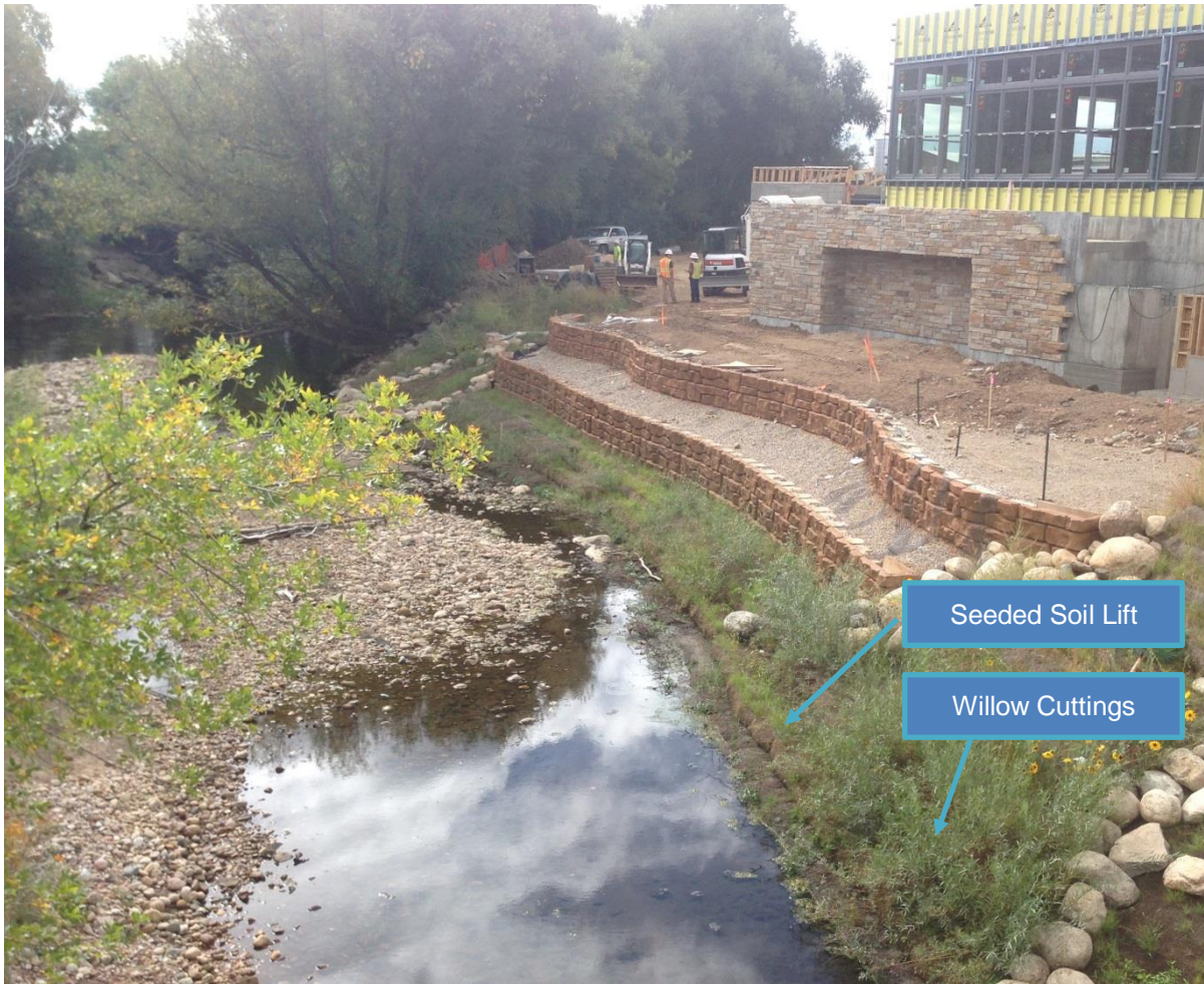
Figure 31. Vegetated soil lifts used to protect high value infrastructure on the Cache la Poudre River, Fort Collins, CO. Two seasons post-construction. From Giordanengo, J. H. Reprinted with permission.
