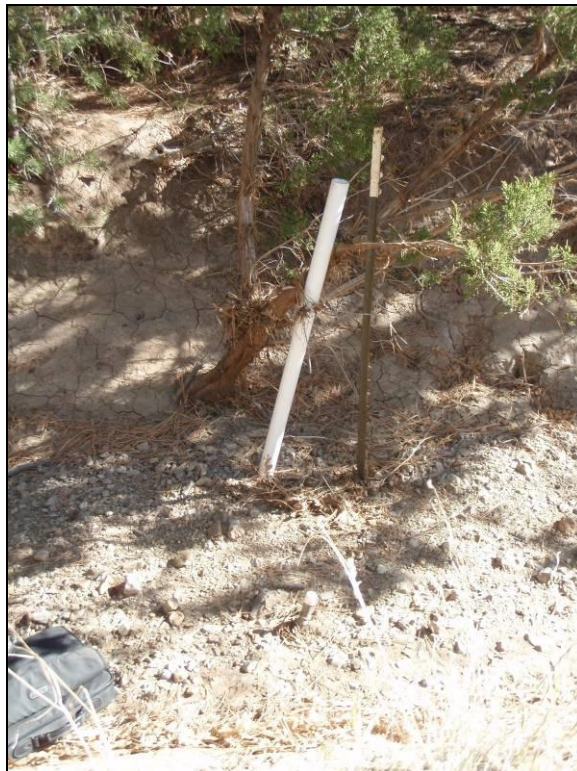
Figure 4.5. Large amounts of deposition and debris accumulation at the Vigil piezometer after a storm event in 2008.
