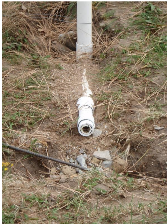
Figure 4.7. Damage to the Chilili piezometer in 2009. Even though the end cap was removed, this piezometer was still able to record flow.
