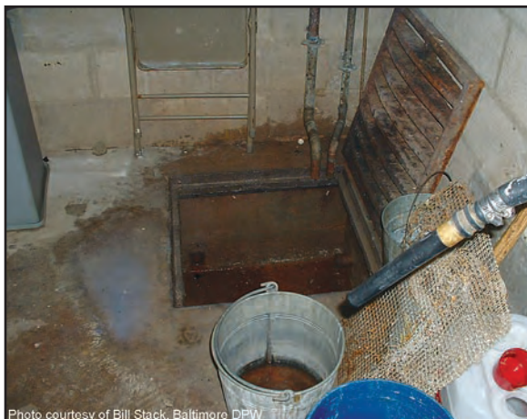
Figure 3: A common industrial cross connection is a floor drain that is illicitly connected to a storm drain
