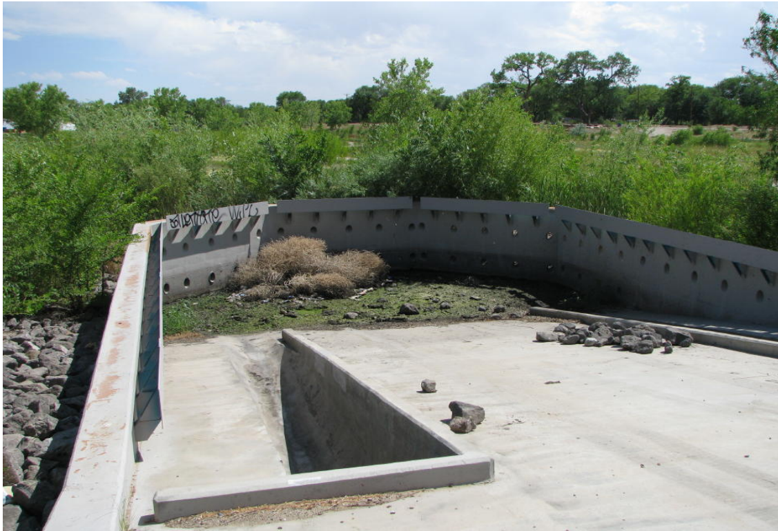
Storm water outlet at Sanchez Farm (simple trash and large debris filtration)
